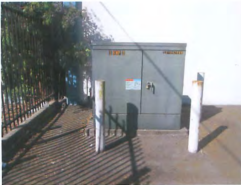
Photo 4: Looking at the electrical box inside the property
