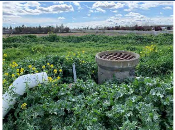
Piping and standpipe near westerly terminus of onsite drainage canal
