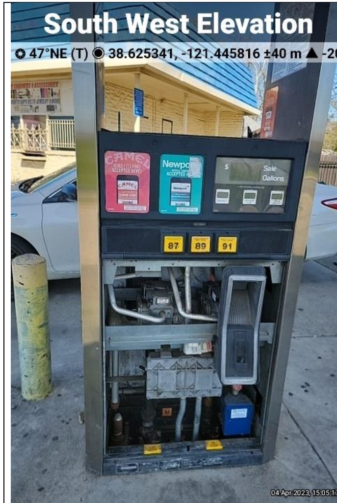
Photo 23 – Fuel dispenser wiring has been removed. View northeast.
