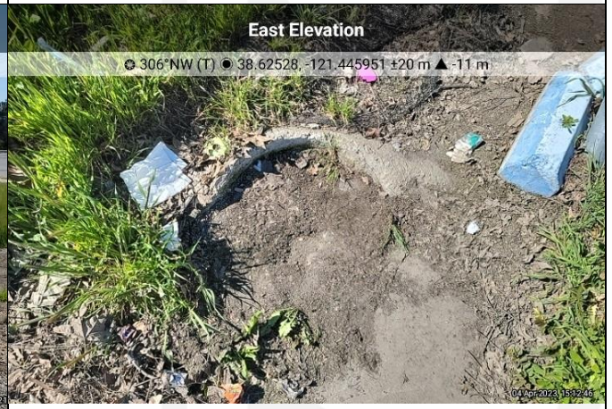
Photo 34 – Round concrete structure within concrete swale at west side may have been associated with storm water drainage but presently filled with soil. View northwest.
