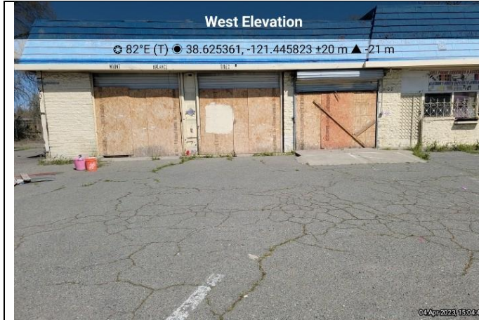
Photo 31 – Bay doors and entry door boarded up for safety. note cracked asphalt. View east.
