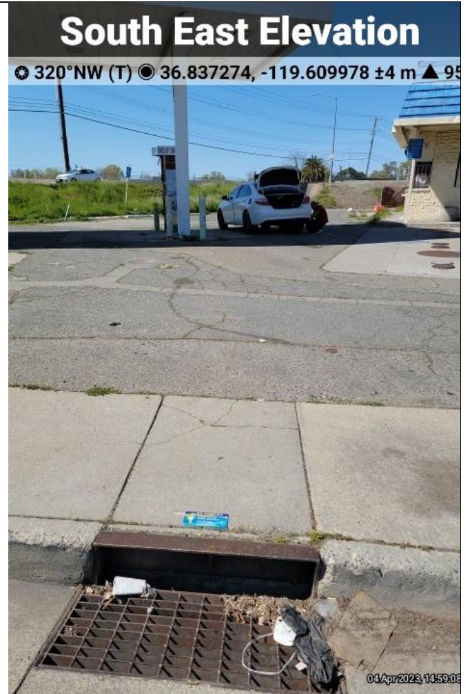
Photo 18 – City of Sacramento MS4 storm drain inlet drains stormwater from the site. View northwest.
