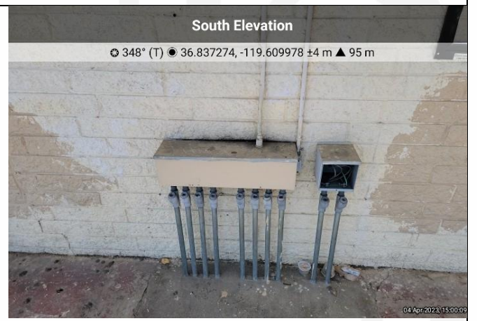
Photo 22 – Fuel dispenser wiring has been removed. View north.
