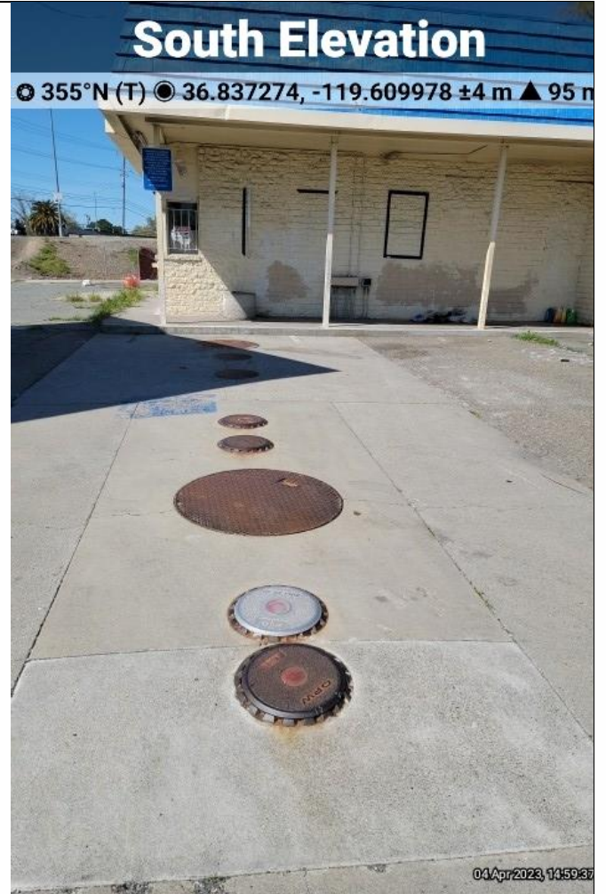
Photo 20 – Tank filling ports. View north.
