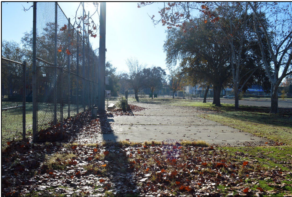
Figure 5. Concrete pad and dugout bench at southwest corner of Renfree Field, view south.
