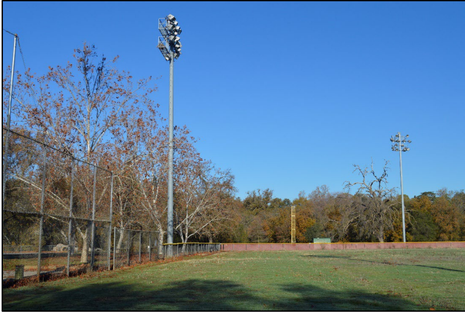
Figure 4. Typical chain-link fencing, lighting, and foul ball post at Renfree Field's left field, view north.
