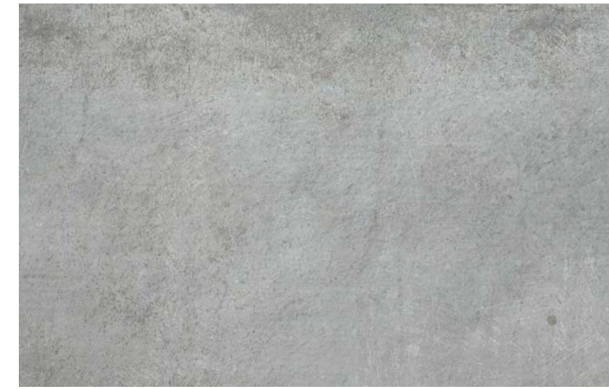
FLOODWALL - EXPOSED CONCRETE AT RIVERSIDE
