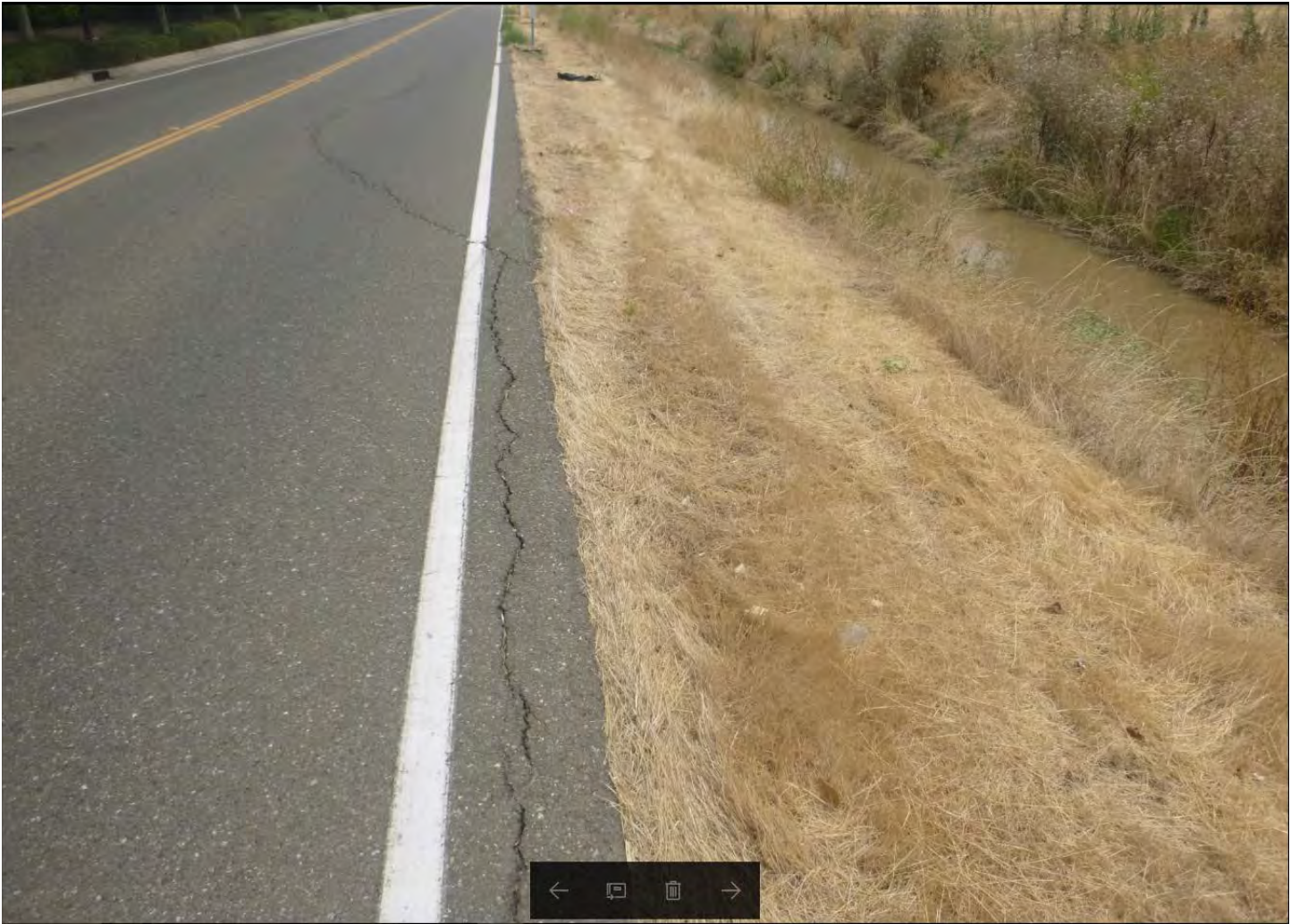
NCD sloughing road.jpg
