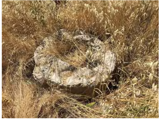
14. View of what appears to be a destroyed water supply well on the adjacent property to the West.
