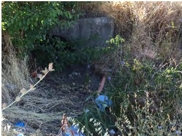
5. Box culvert within the drainage ditch in the north-eastern most portion of the Subject Property.
