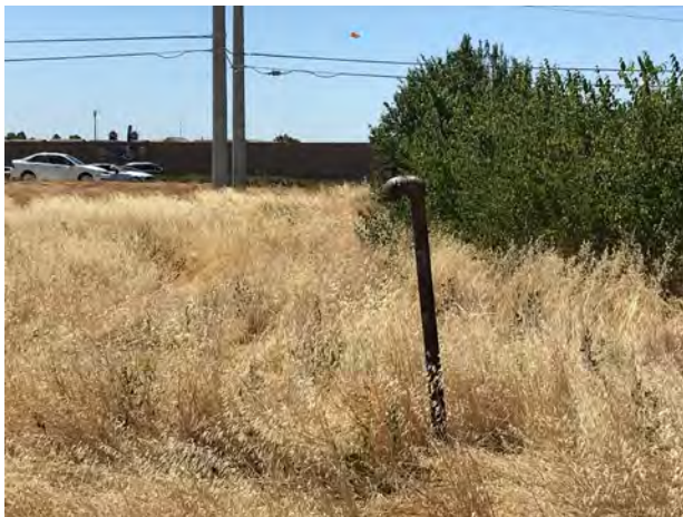
15. What appears to be an unidentified vent pipe along the western perimeter of the Subject Property.
