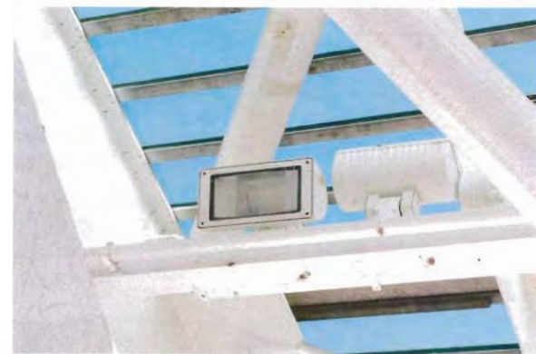
Photo 7. View of the Sundial Bridge under-deck lights, with one facing down towards the river and one facing up towards the bridge deck.
