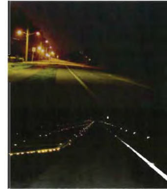
Figure 4. An example of embedded roadway lighting from Boca Raton, Florida. In the top view, the streetlights are visible from the sea turtle nesting beach, while the embedded lights in the lower view are not visible from the beach (Bertolotti and Salmon 2005). Figure reprinted from "Protecting Sea Turtles from Artificial Night Lighting at Florida's Oceanic Beaches" by Michael Salmon. Found in Ecological Consequences of Artificial Night Lighting by Catherine Rich and Travis Longcore, eds. Copyright © 2006 Island Press. Reproduced by permission of Island Press, Washington, D.C.
