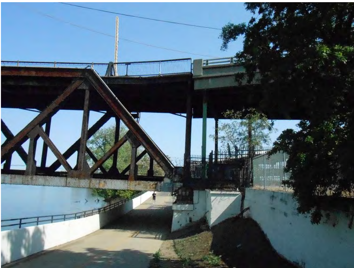
Photograph 3. Showing terminus of bridge on Sacramento County side. The bridge terminates at the end of the truss and the abutment, shown to the right of the walkway near the center of the photograph.
