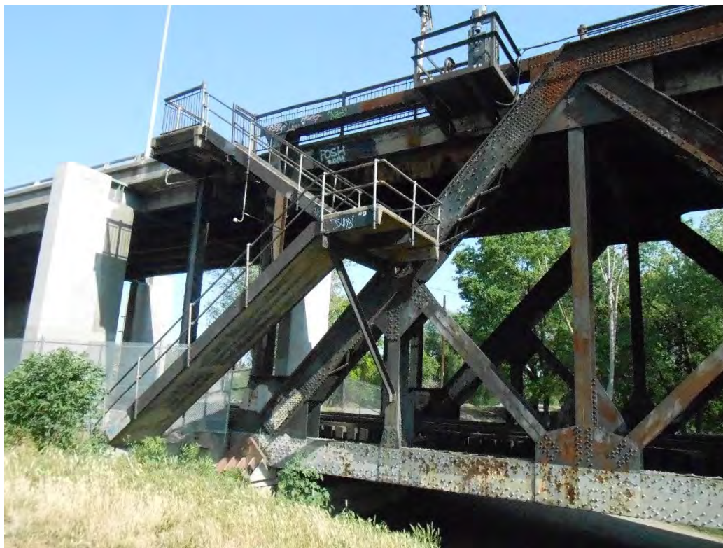
Photograph 4. Showing terminus of bridge on Yolo County side. The bridge terminates at the end of the truss, shown near the center of the photograph. The pedestrian stair is a modification, partially attached to the 1911 structure.
