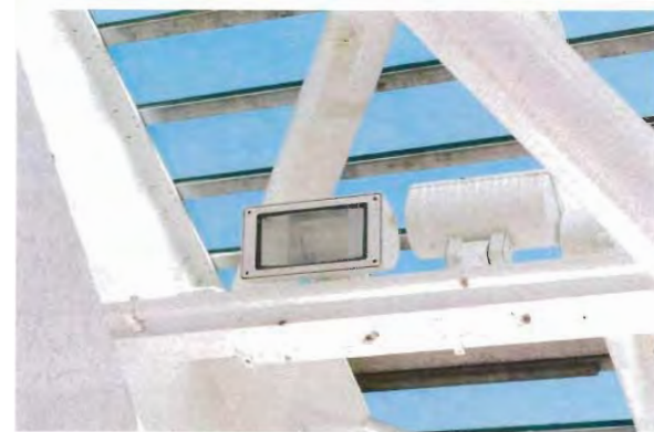
Photo 7. View of the Sundial Bridge under-deck lights, with one facing down towards the river and one facing up towards the bridge deck.
