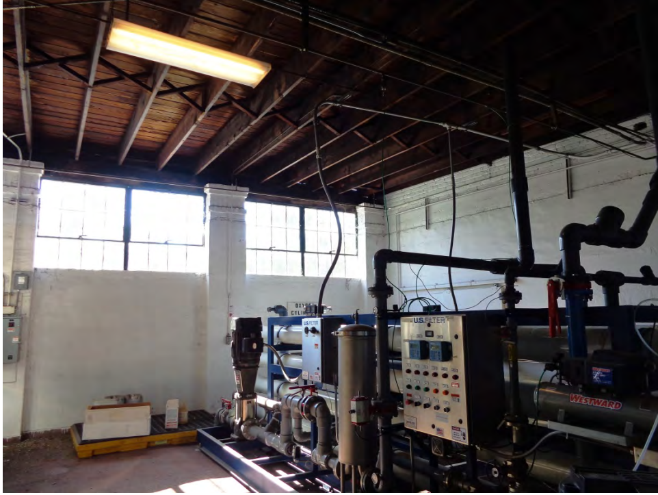
Pump Room (southwest)
