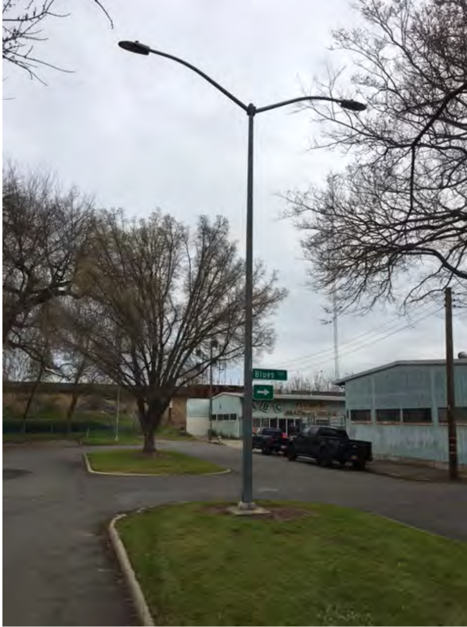
DUAL MAST ARM STYLE STREET LIGHT
