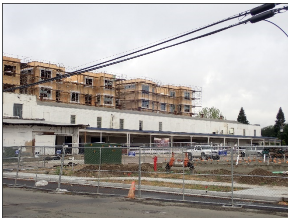
Photograph 6. P-47-03382 Farmers Market building segment adjacent to 5 th St. (#3a) view to southwest)
