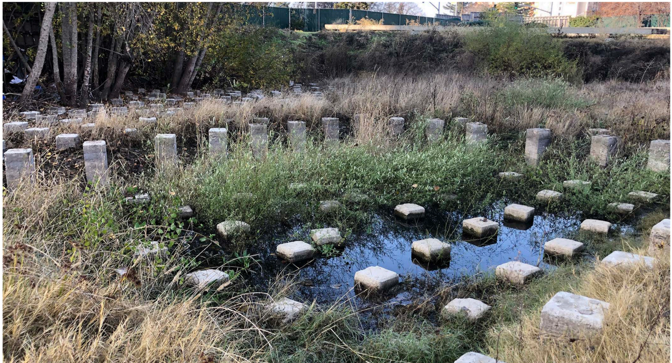
Viewpoint 2: Remnants of foundational piles in the southeastern quadrant of the project site from a previous uncompleted project. View facing northwest.
