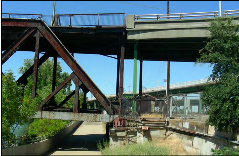
Photograph 17: I Street Bridge meets I Street Viaduct and J Street Viaduct, camera facing north, July 2007.
