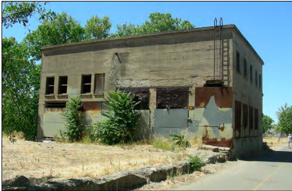
Photograph 14: Remnant (pumphouse) of former Pioneer / Sperry Mill, south side, camera facing northwest, July 2007.
