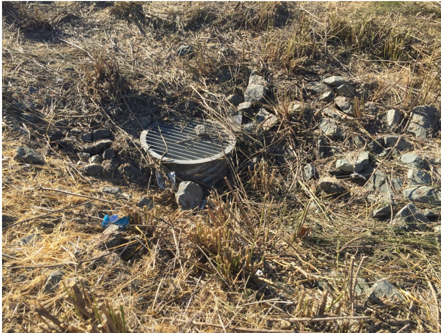
View of drainage intake within the feature during dry season, after vegetation has been cleared (July 27, 2016)
