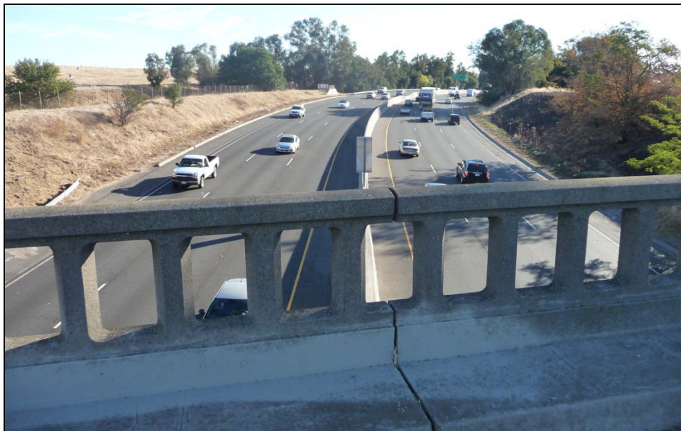
Photograph 2: A Street OC railing and view of freeway. B Street Underpass floodgates are in the background, 8/16/13.
