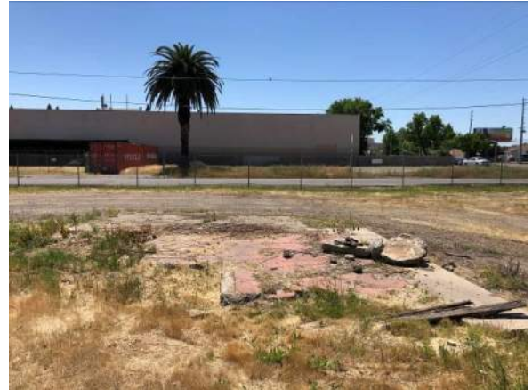
Photo #8 View of concrete debris, located on the south-southeastern portion of the site in the former location of warehouse.
