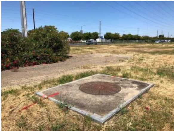
Photo #9 View of SMUD utility manhole, located on the southwestern portion of the site.
