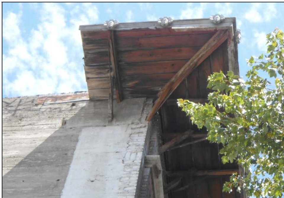
Photograph 5: Detail view of cornice substructure at southwest corner that projects over the property line, July 16, 2014 (ESA).
