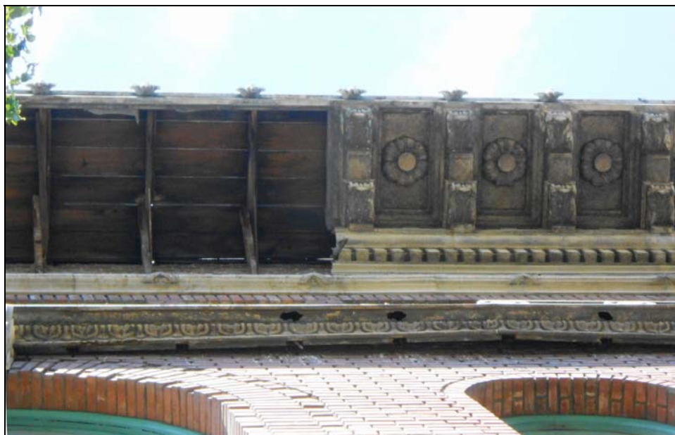
Photograph 6: Detail view of missing cornice and original cornice in place near southwest corner, July 16, 2014 (ESA).
