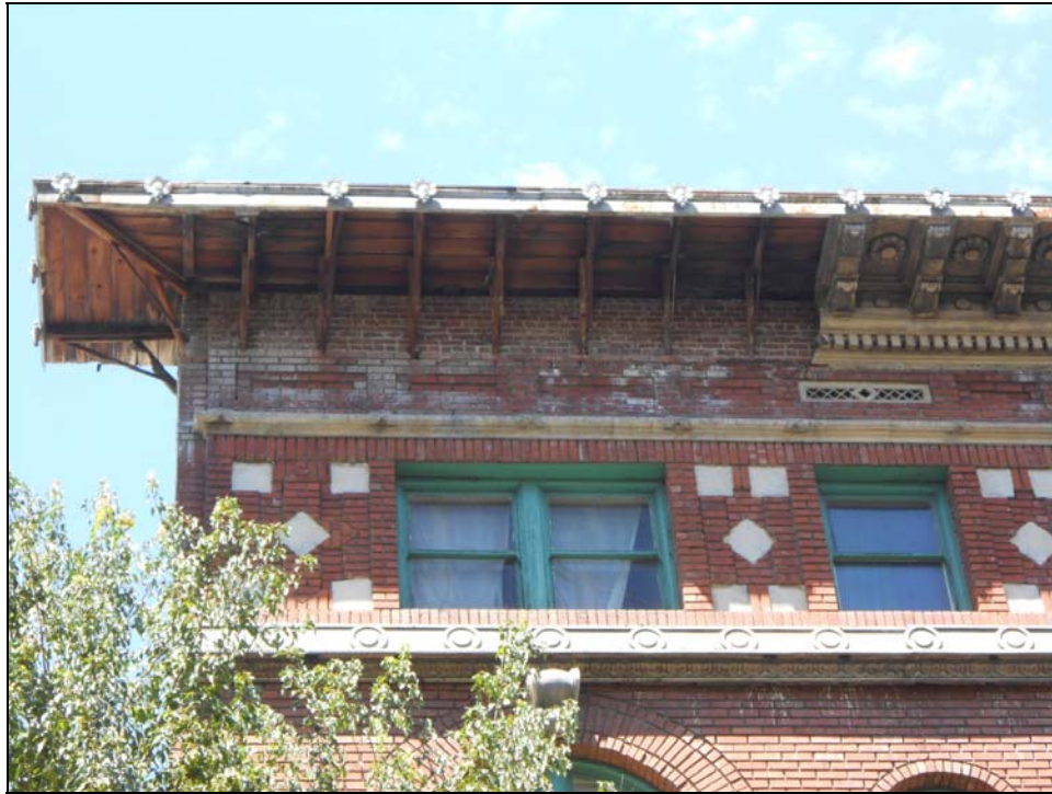
Photograph 4: Missing cornice elements at southwest corner, camera facing north, July 16, 2014 (ESA).
