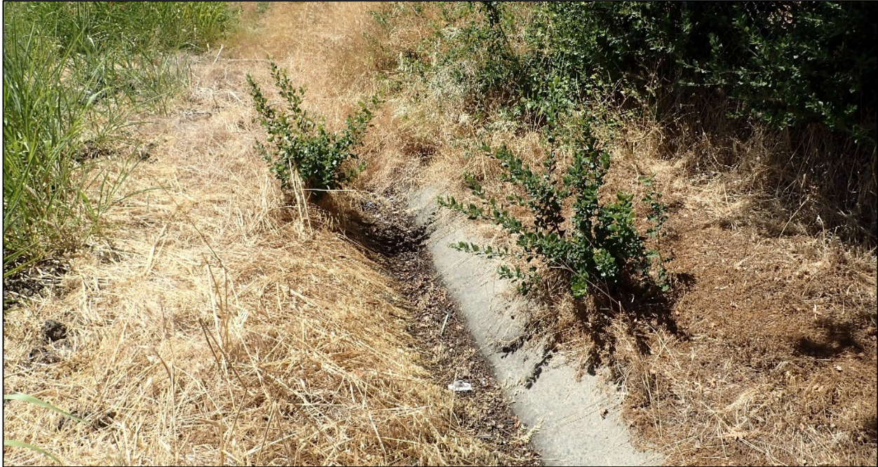
Photograph 5. The image shows the concrete drainage ditch within the northwestern portion border of the Study Area. View facing southwest. Photograph taken July 7, 2017.
