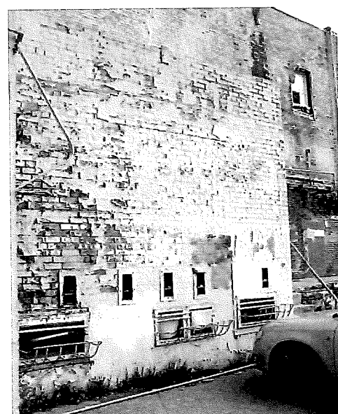
View northeast of south façade of ice dispensing facility (Accession 08-8007-DIG-1-21, Feb. 24, 2009)
