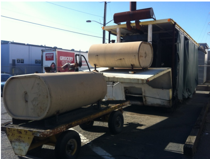
11. View of a diesel generator AST and portable diesel AST along the north boundary of the site
