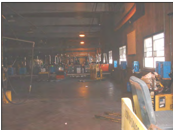
Photo 5 – Battery charging room
