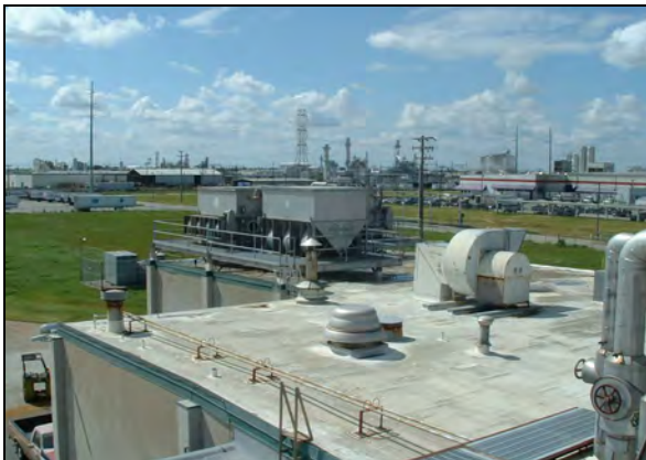
Photo 11 – Equipment on top of refrigeration room
