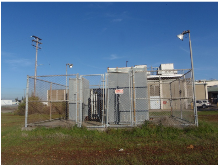
7. View of a property owned pad-mounted transformer on the southwest side of the subject property
