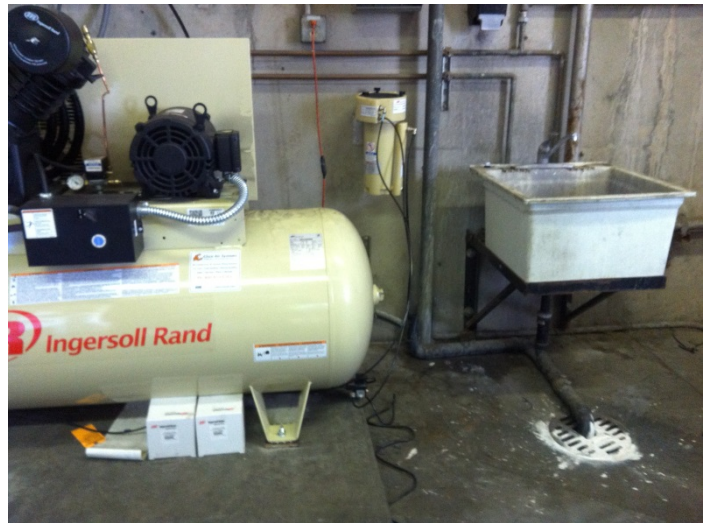
52. View of a new air compressor with an oil/water separator system located on the wall; water from the separator system leads directly to the floor drain/sewer system
