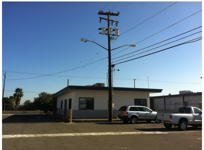
4. View of three property owned pole-mounted transformers adjacent to the west of one of the two office structures on the northeast side of the property
