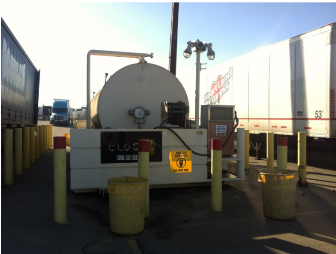
15. View of one of three 12,000-gallon empty (formerly containing diesel) ASTs in secondary containment
