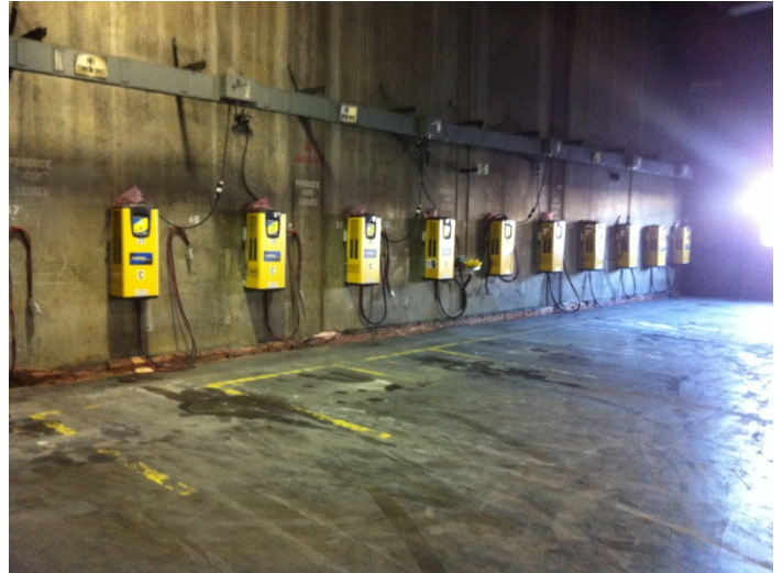
46. View of the battery charging room on the north side of the main subject property building
