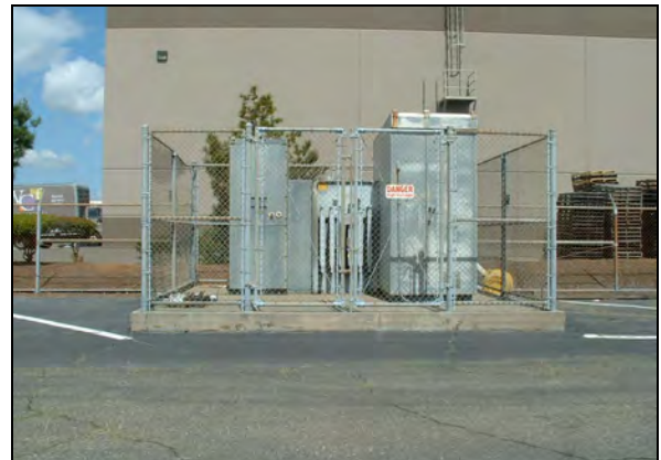
Photo 12 – A pad-mounted transformer on the subject property
