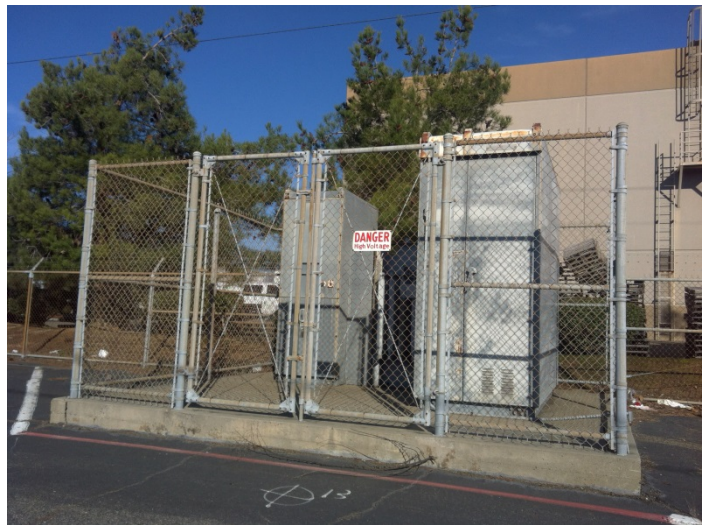
8. View of a property owned pad-mounted transformer located along the north boundary of the site
