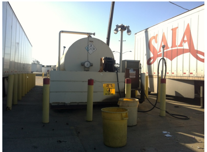
16. View of one of three 12,000-gallon empty (formerly containing diesel) ASTs in secondary containment
