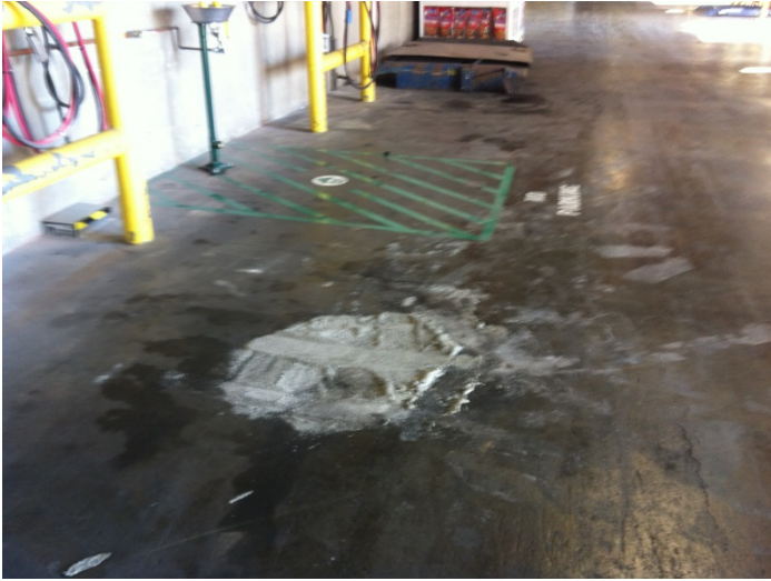
41. View of a stain observed in the loading dock area of the main subject property building
