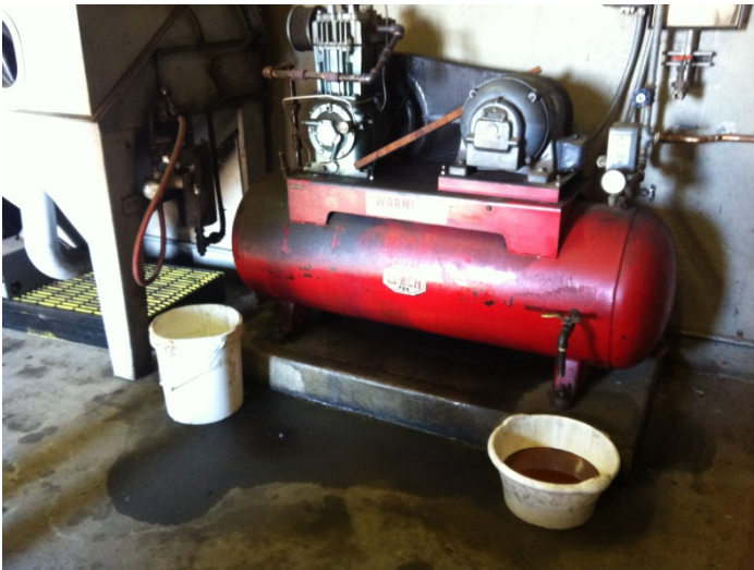
51. View of a decommissioned air compressor with staining observed in the vicinity and an open catch bin containing oily fluid
