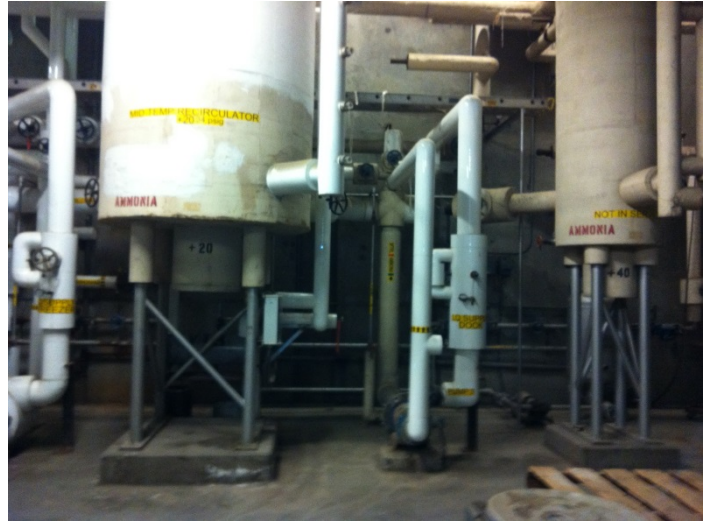
54. View of the ammonia refrigeration equipment observed in the ammonia refrigeration room
