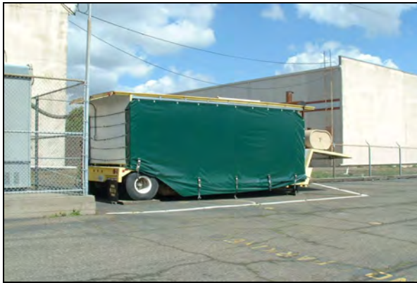
Photo 13 – The emergency generator on the subject property
