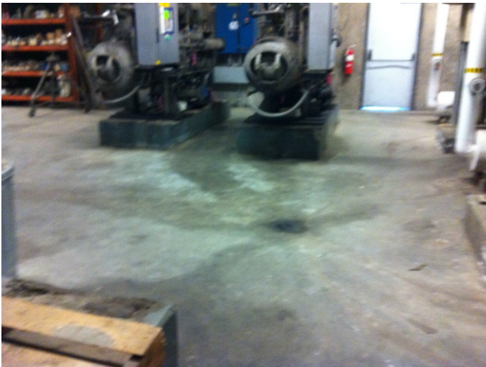
55. View of a drain observed in the ammonia refrigeration room with minor staining in the vicinity
