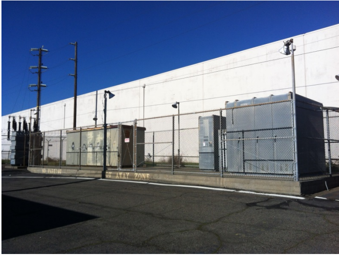
9. View of one SMUD owned substation transformer (far left) and two property owned pad-mounted transformers along the north boundary of the site
