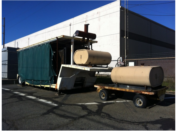
10. View of a diesel generator AST and portable diesel AST along the north boundary of the site
