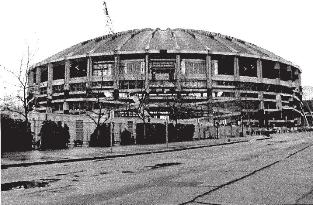
The Kingdome, Seattle, WA. March 2000. This photograph was taken immediately prior to the implosion, during the intentional weakening of the building frame to prepare for the implosion. Photo by Charlene Roise.
