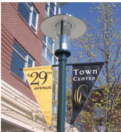
Pole-mounted light fixture.
