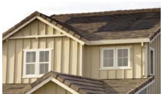
Building integrated photovoltaic panels.
