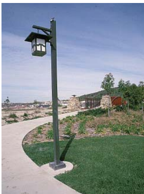
Pole-mounted site lighting fixture
