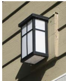
Wall-mounted light fixture
