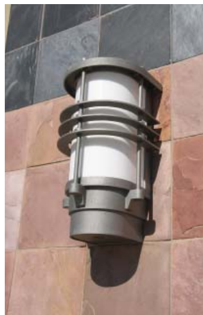
Specialized lighting is appropriate for entries.
