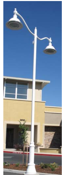
Pole-mounted light fixture.
