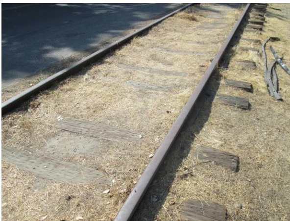
Image 3: Walnut Grove Branch Line Railroad, detail view of typical conditions, near 27 th Avenue. Source: GPA Consulting, 2017.
