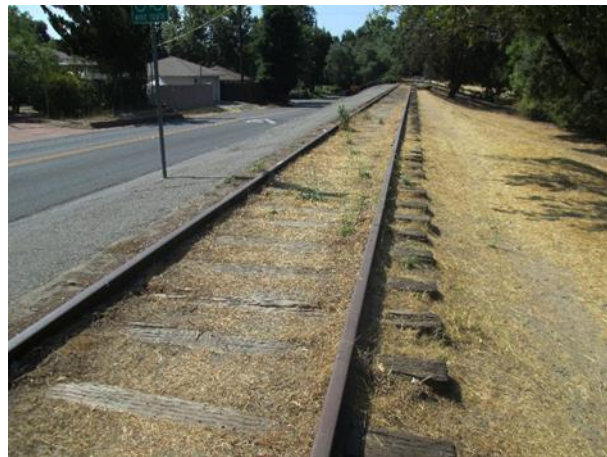
Image 2: Walnut Grove Branch Line Railroad, detail view of typical conditions, along 27 th Avenue. Source: GPA Consulting, 2017.
