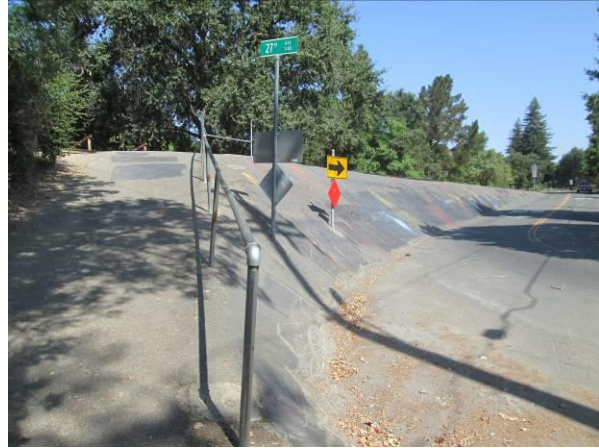
Image 6: Walnut Grove Branch Line Railroad, view looking northwest from 27 th Avenue. Source: GPA Consulting, 2017.
