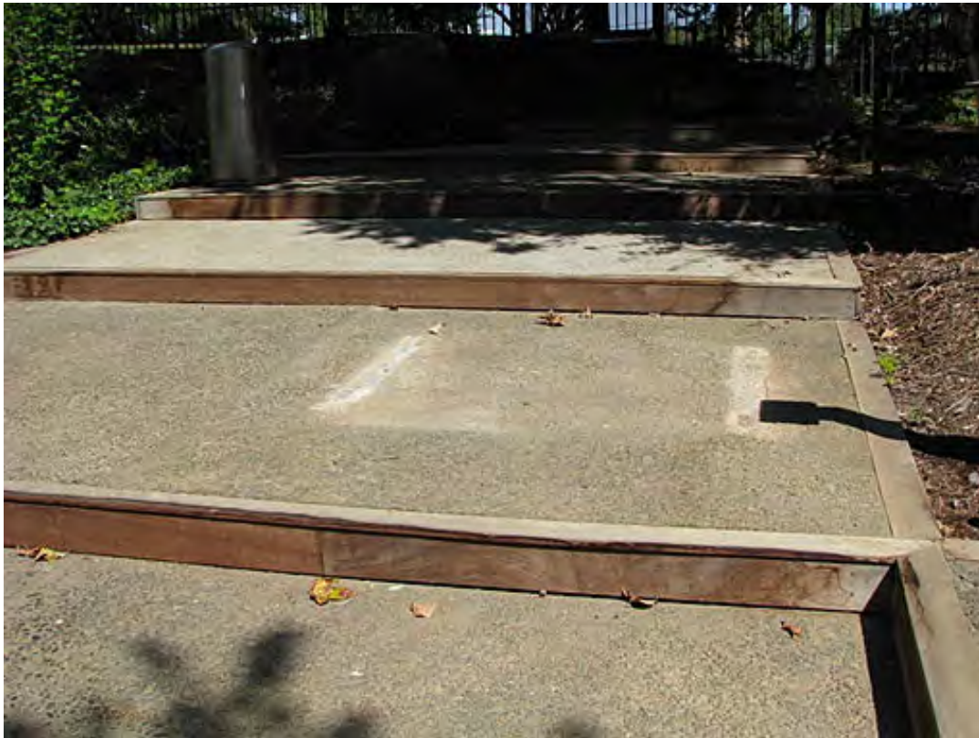
PHOTOGRAPH 70: Cafeteria terracing showing former location of missing site furnishings.
