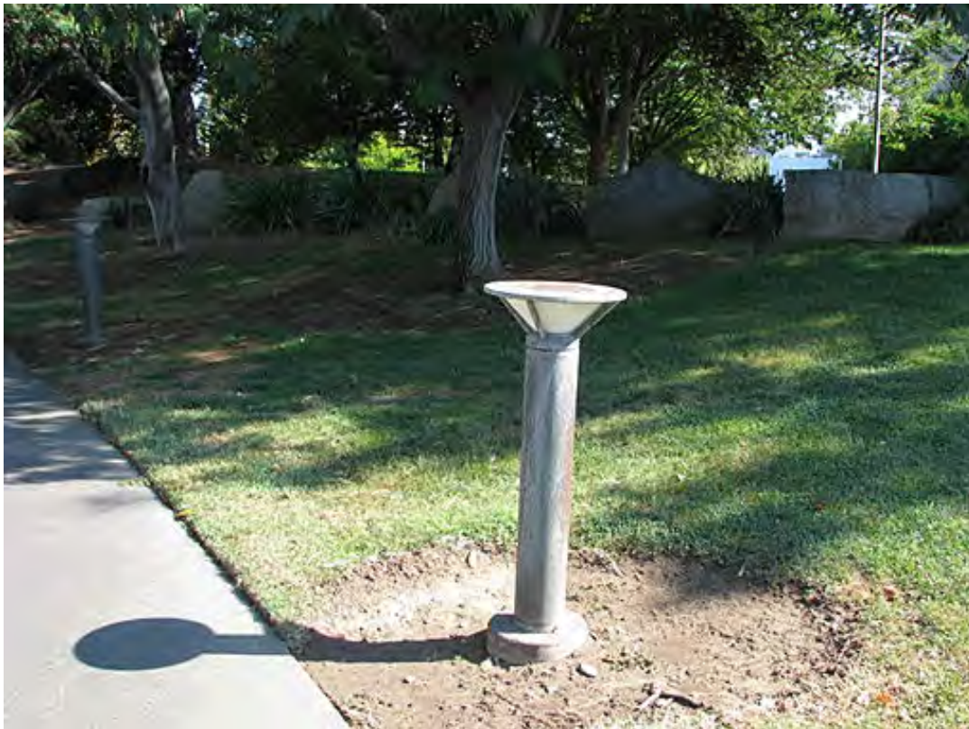
PHOTOGRAPH 13: Typical bollard light.
