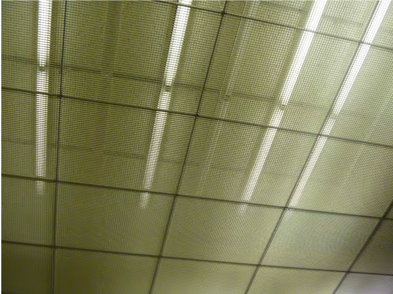
Figure 16. Original luminous ceiling.
