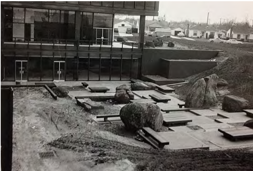
PHOTOGRAPH 2: March 24, 1960 construction of the cafeteria terrace showing the grading, retaining walls, new boulders, terracing, and site furnishings behind the south wing of the building.
