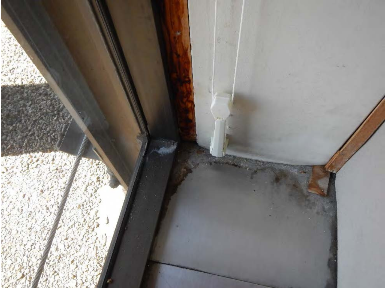
Figure 27. Water damage at metal duct cover, fourth floor of south wing.
