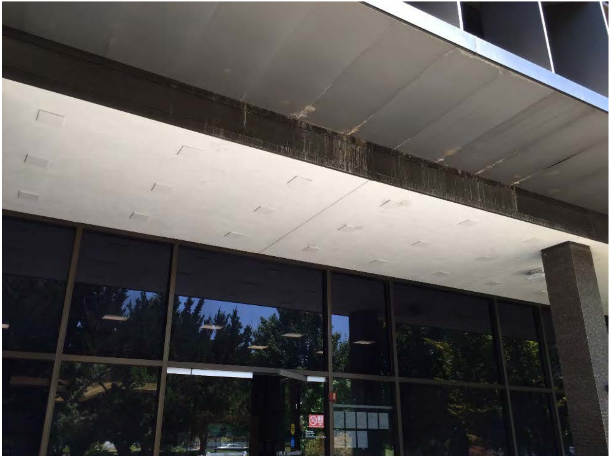
Figure 12. White streaking at spandrel, under brise soleil.
