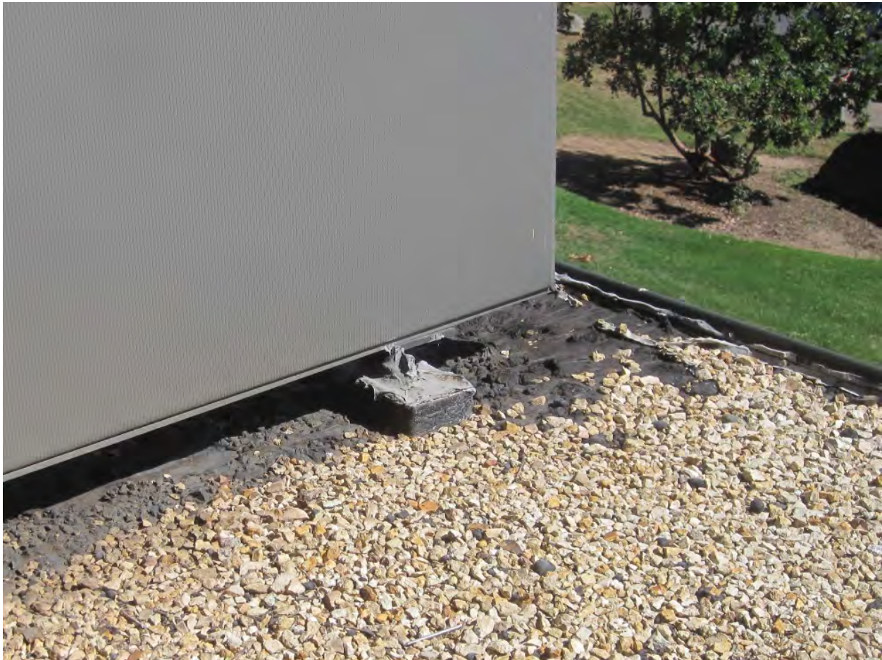
Figure 15. Gravel-surfaced coal tar roof and gravel stop at surface of typical cantilevered ledge.
