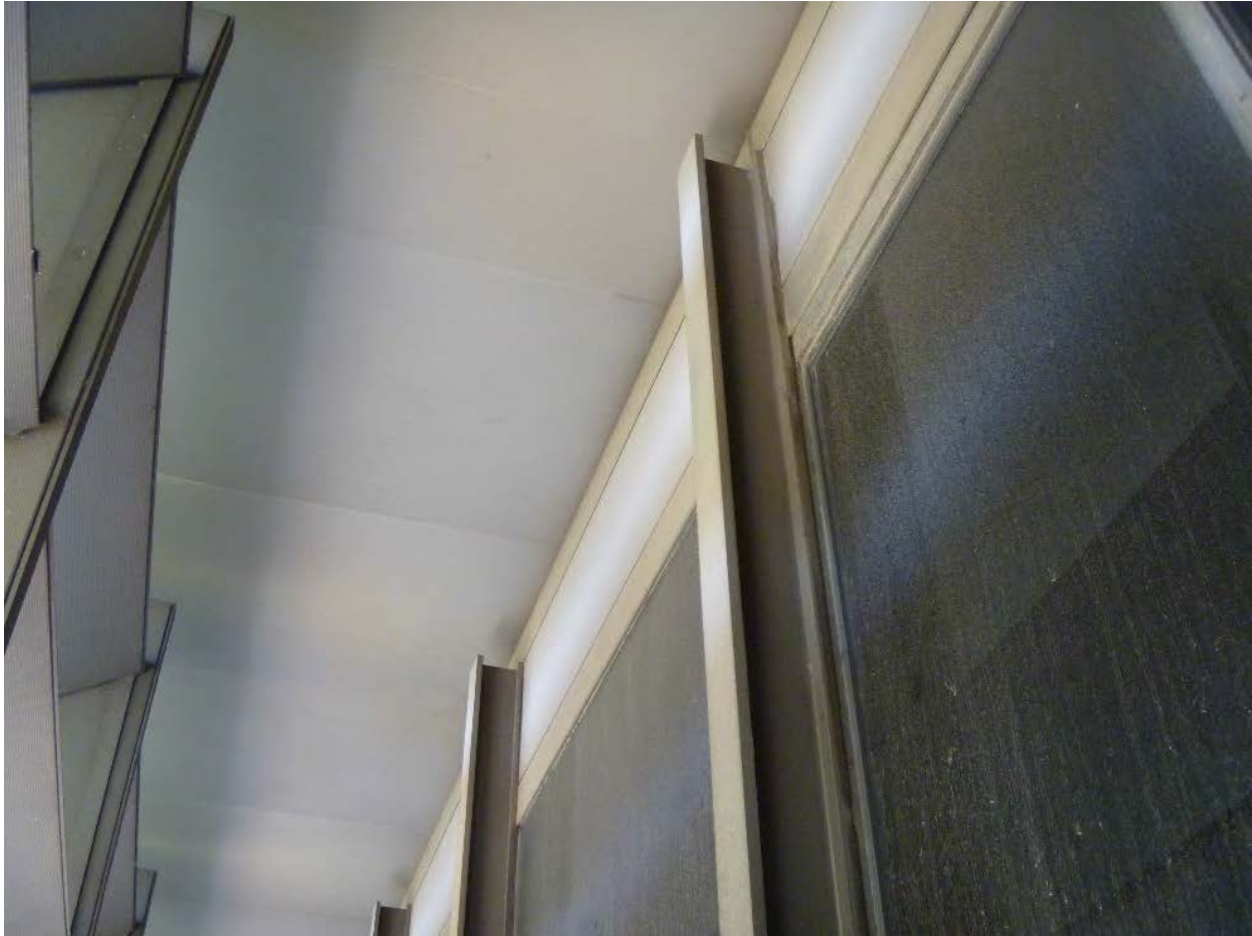
Figure 10. Upper-floor glazing attached to vertical I-mullions.
