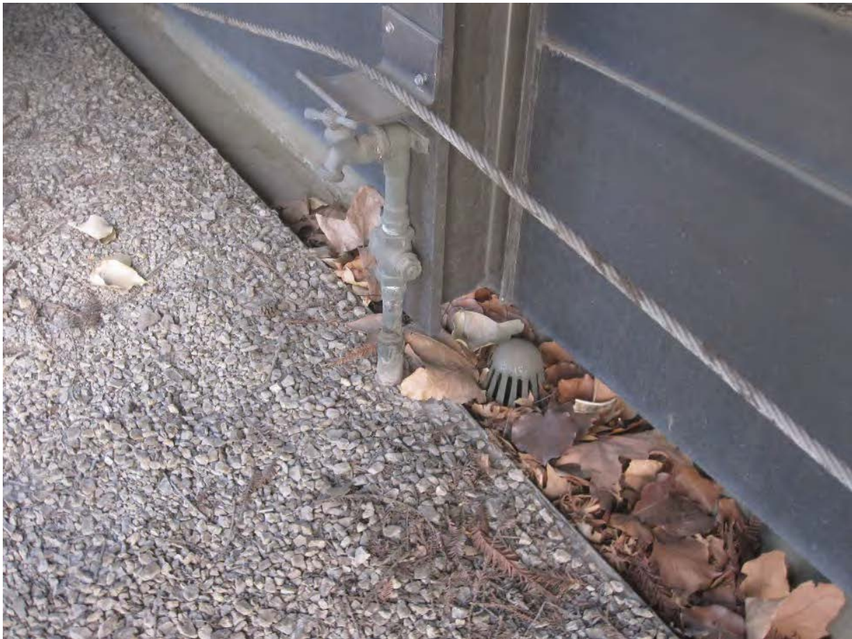
Figure 14. Internal gutter full of debris at cantilevered ledge.
