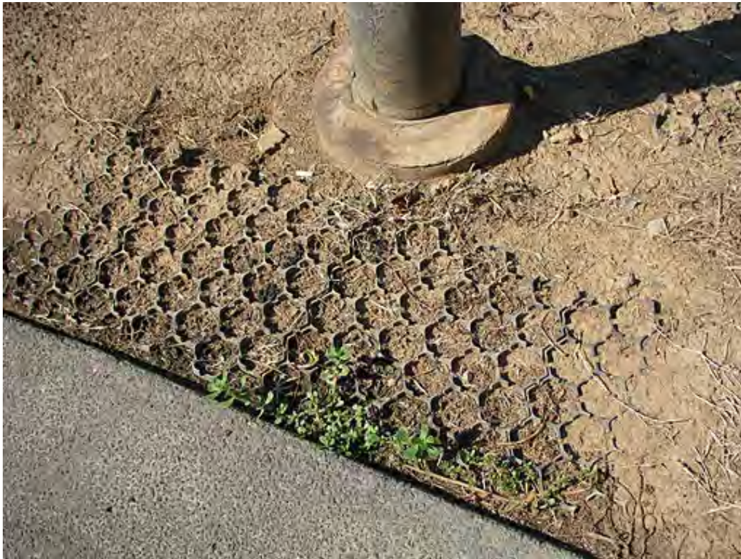
PHOTOGRAPH 20: Erosion and erosion control matting along path.
