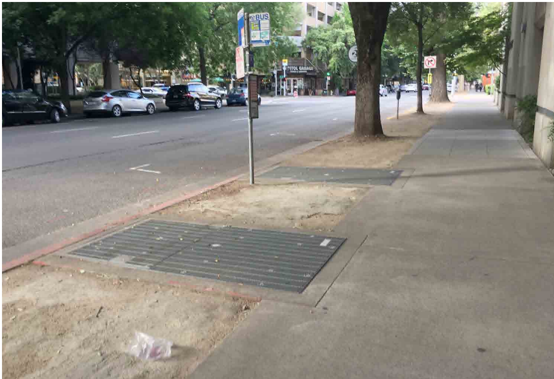
Photo No. 18 Vaulted transformers owned by SMUD adjacent to the administrative building at 1530 15th Street
