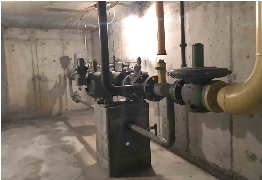
Photo No. 8 Gas main in vented vault in basement
