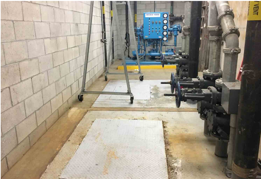
Photo No. 10 Water booster pump, dewatering and sewer sumps
