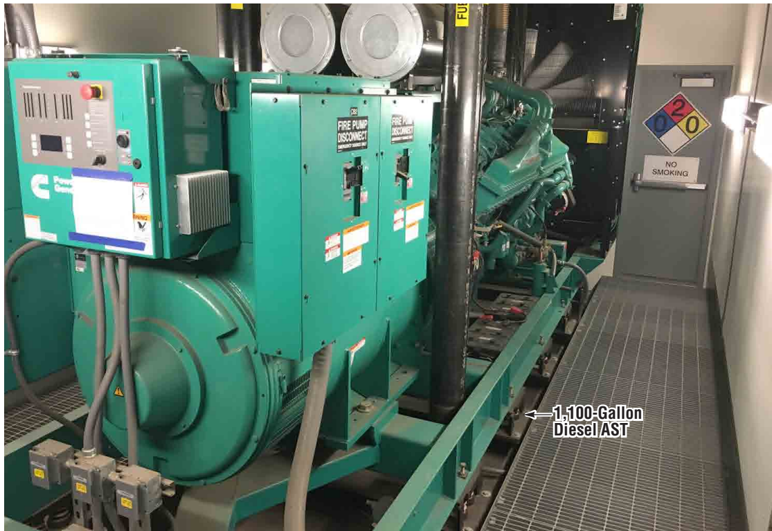
Photo No. 21 Generator over 1,100-gallon diesel AST
