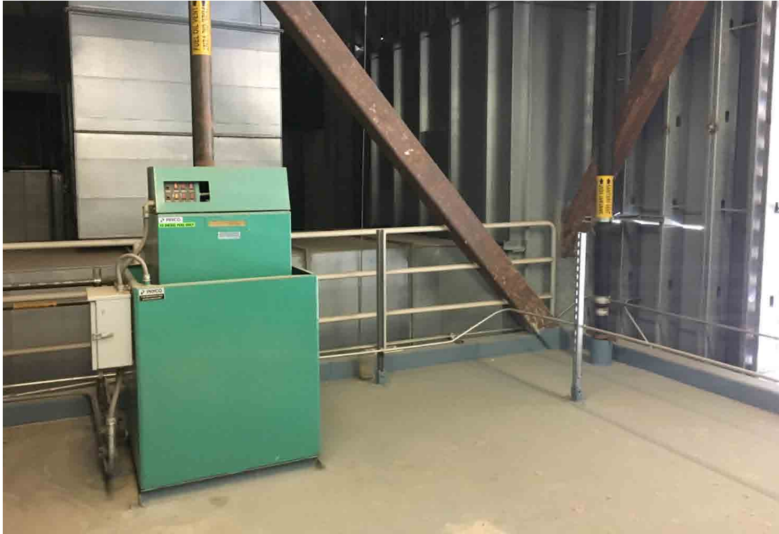
Photo No. 15 Empty and disconnected diesel holding tank for the formerly utilized generator
