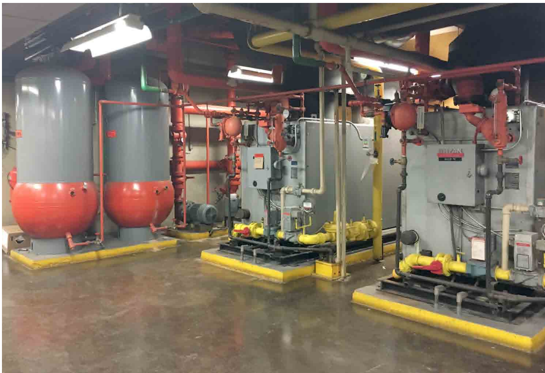
Photo No. 6 Boilers and holding tanks in the basement, Central Plant
