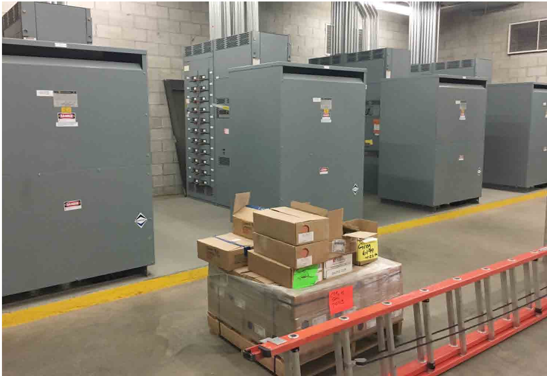
Photo No. 7 Dry-type transformers in basement
