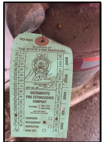
Figure 12: Fire Extinguisher Last Inspected in 2003
