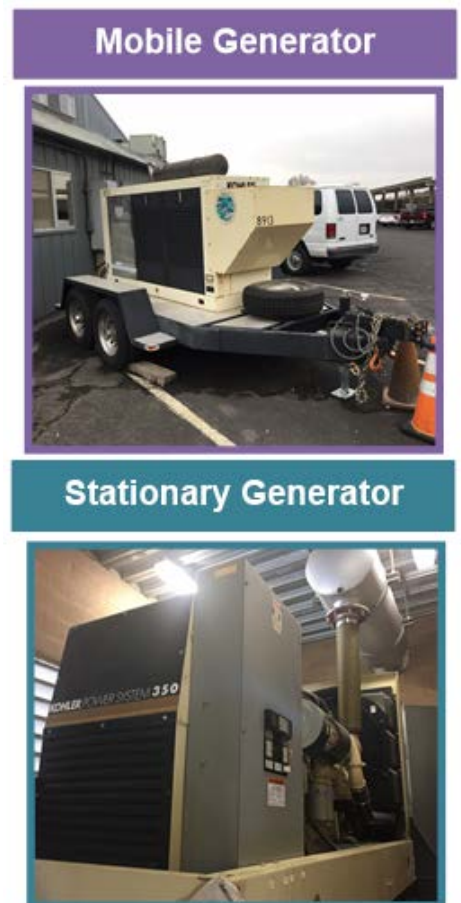
Source: Mobile Generator photograph provided by the Fleet Management Division and Stationary Generator photograph taken by audit staff.
